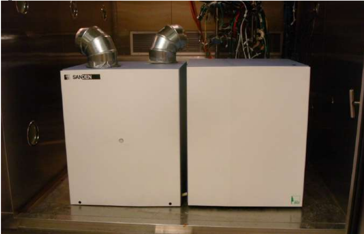
Figure 1. HPWH Test Unit Installed Inside Thermal Chamber
